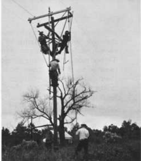
A Santee crew, working while the lines are hot, installs a new cross arm on a pole.
