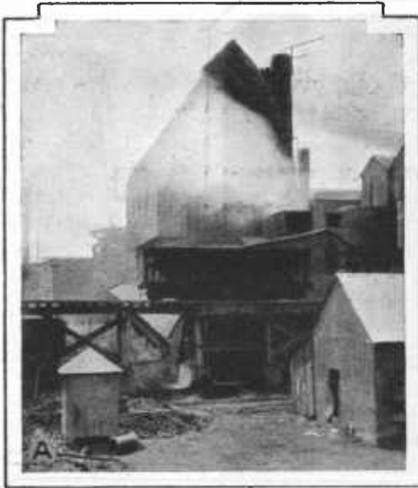
A, Cottrell precipitator installed at one of the cement plants for the collection of potash-bearing dust. Precipitator not operating; fumes escaping.
