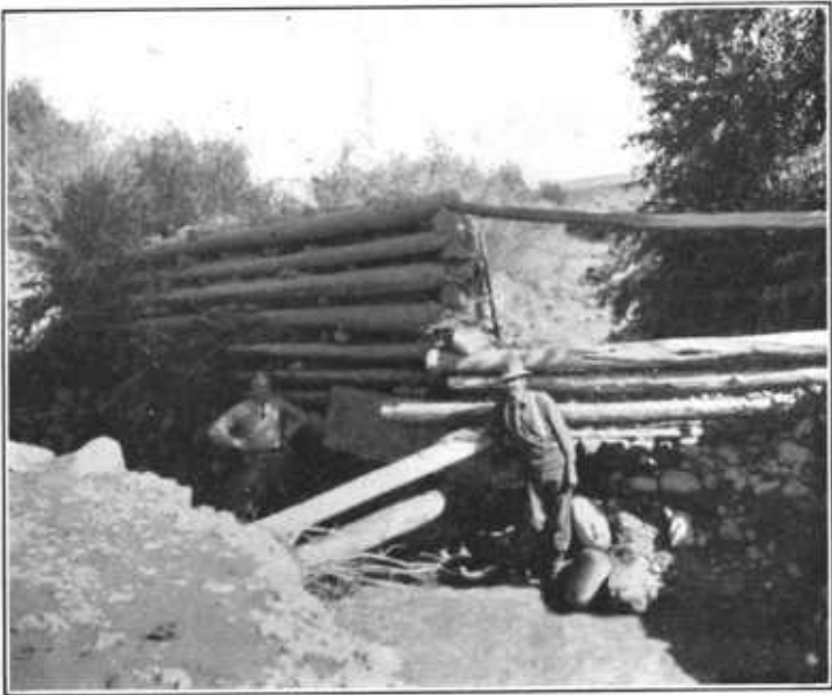
FIG. 1.—IMPORTANT IRRIGATING DITCH AND LATERAL LESS THAN ONE MILE FROM BUSINESS SECTION OF EPHRAIM CITY, UTAH, BADLY DAMAGED BY THE FLOOD OF AUGUST 24, 1912.
