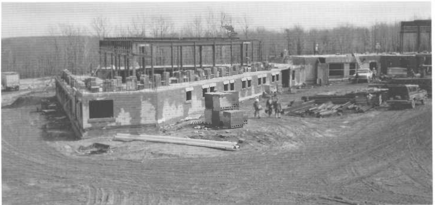
Federal Correctional Institution under construction in Schuylkill, PA in 1990 now houses inmates.
