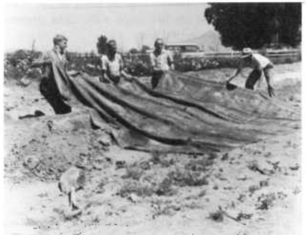
FIGURE 15.—A section of liner, composed of several widths seamed together on the bank, is pulled into place.
