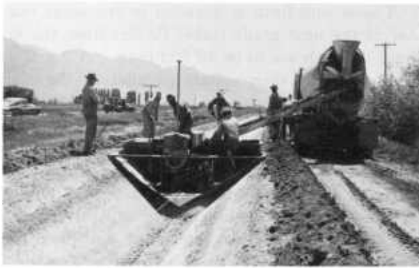
FIGURE 4.—Front end of slip form, showing winch and cable attached to anchor ahead for advancing slip form.
