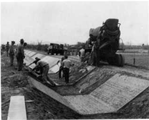
FIGURE 8.—Concrete lining being constructed by the panel method: Panel in foreground has just been screeded, a 10-foot space is skipped, and another panel is in the process of being placed.
