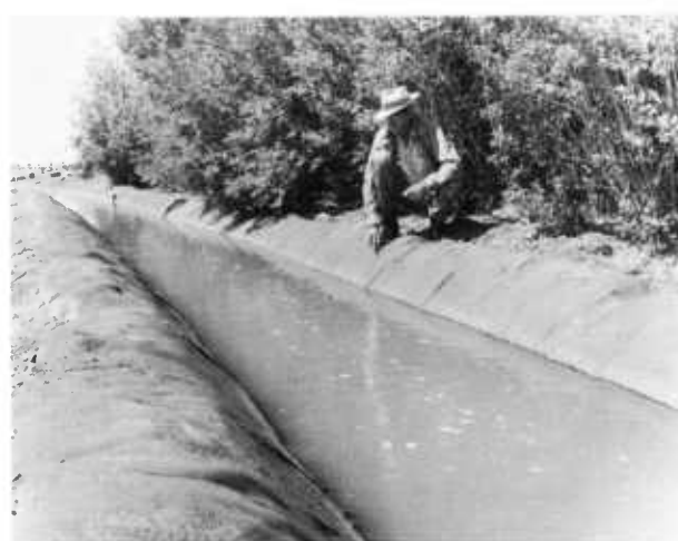
FIGURE 18.—Lined ditch in operation.
