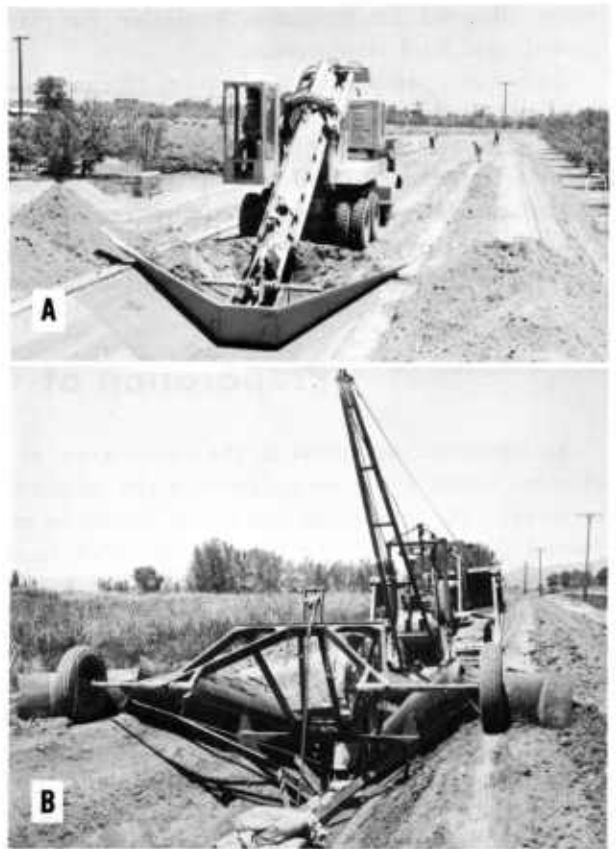
FIGURE 2.—A, A Gradall excavating a small lateral; B, plow used to excavate field ditch in preparation for lining with slip-formed concrete.
