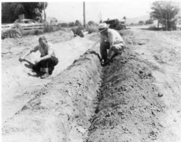
FIGURE 16.—Ditch prepared to receive lining. Note trench in berm for anchoring lining.
