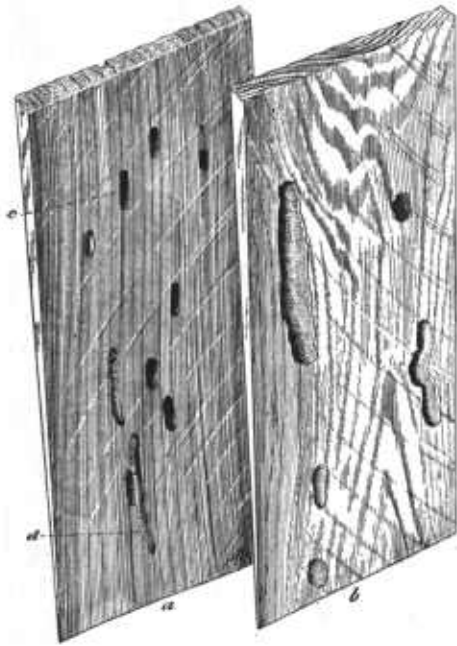
FIG. 2.—Western red cedar shingles badly damaged by larval mines of Trachykele blondelli : a , Quarter-sawn shingle showing both cross and longitudinal sections, c , d , of the larval mines; b , bastard-sawn shingle showing same
