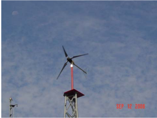
Fig.2. SWWP Whisper 100 Wind Turbine. (Bushland, TX).
