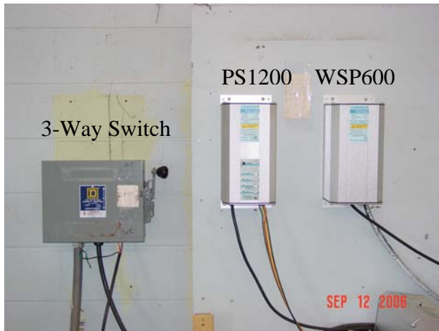
Fig.4. 3-Way Switch and Controllers Used on Wind Powered Water Pumping System. (Bushland, TX).
